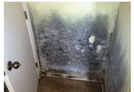
Mold damage on wood frame construction pictured above.
