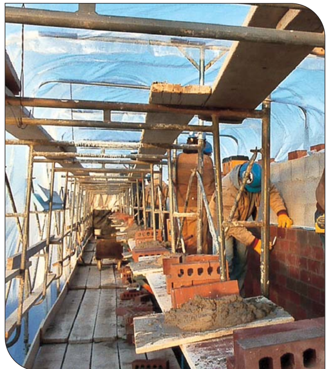
Fig. 12. Enclosure and heating of a work area protects materials, workers, and installed masonry from severe weather. (IMG12508)
