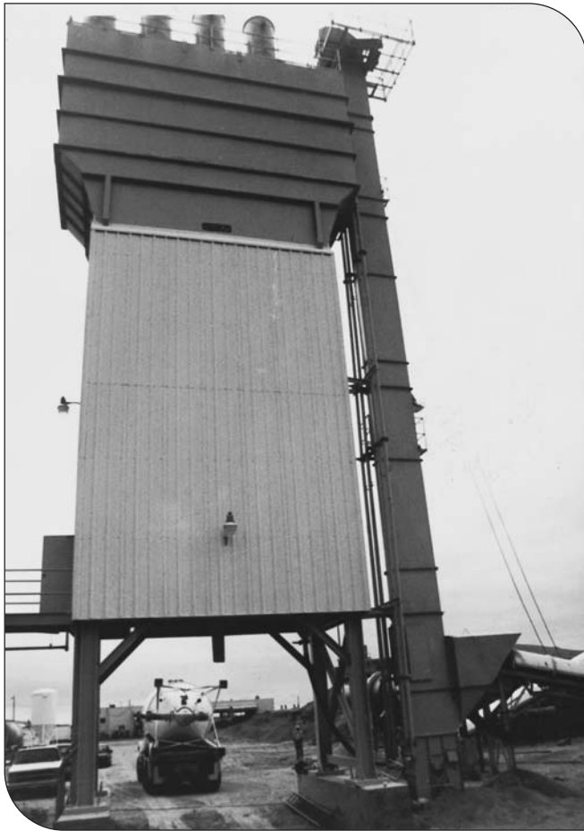
Fig. 13. The storage bin/batcher at this central plant stores individual mortar ingredients (masonry cement, portland cement, lime, and sand) in separate compartments. The computer controlled plant batches the dry ingredients by weight and dry blends them prior to discharge into the silos. (IMG14081)
