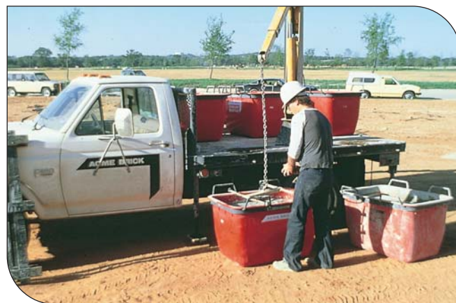
Fig. 15. Extended life, or ready-mixed, mortar is often delivered in mortar containers (tubs) or a flatbed truck. The mortar-filled containers are unloaded and left at the jobsite. (IMG14082)
