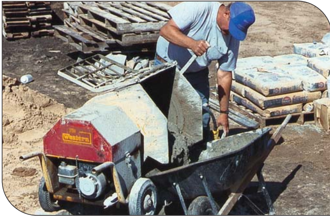
Fig. 9. For best results, the mortar should be mixed with a power mixer. (IMG14592)
