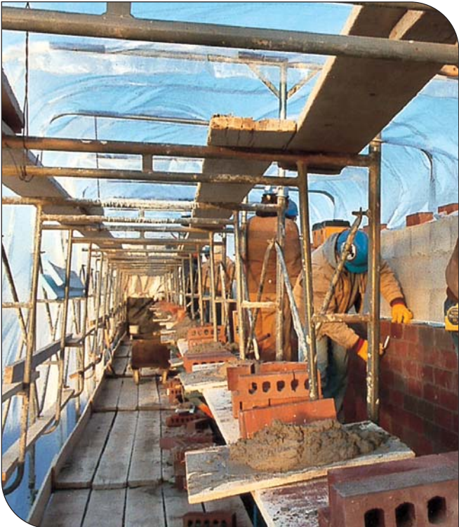
Fig. 12. Enclosure and heating of a work area protects materials, workers, and installed masonry from severe weather. (IMG12508)
